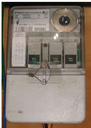
Modern Enermet R03 ripple relay (with Telenerg coding)
