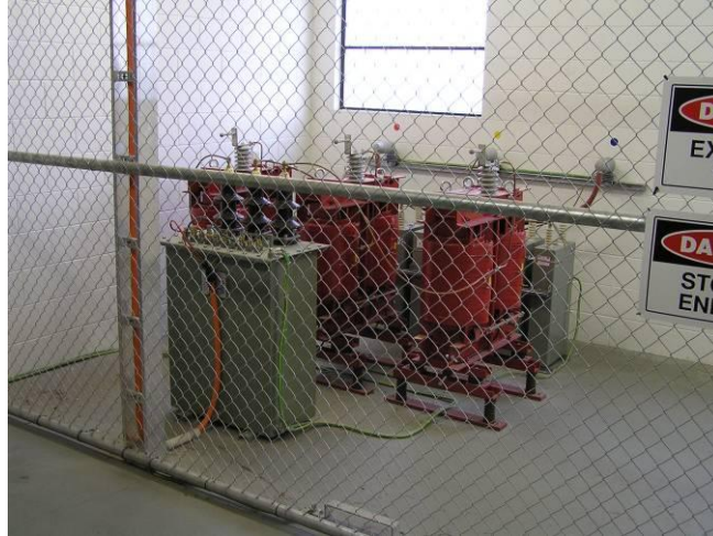
Orion's 11kV ripple injector at the Heathcote district substation
